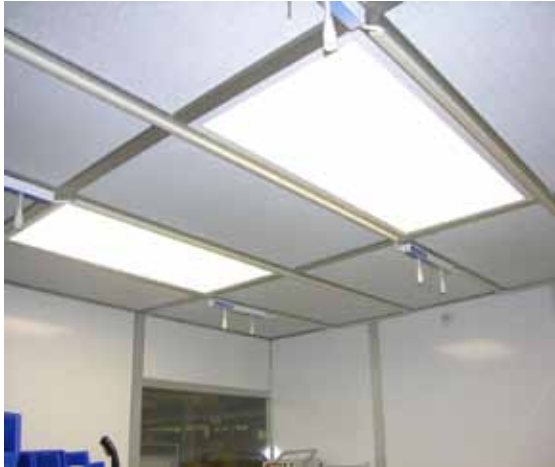
Room System Ionization (Ceiling Grid)
